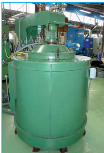
Steam tempering plant
